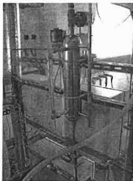
b). Workless boiler feeding system
