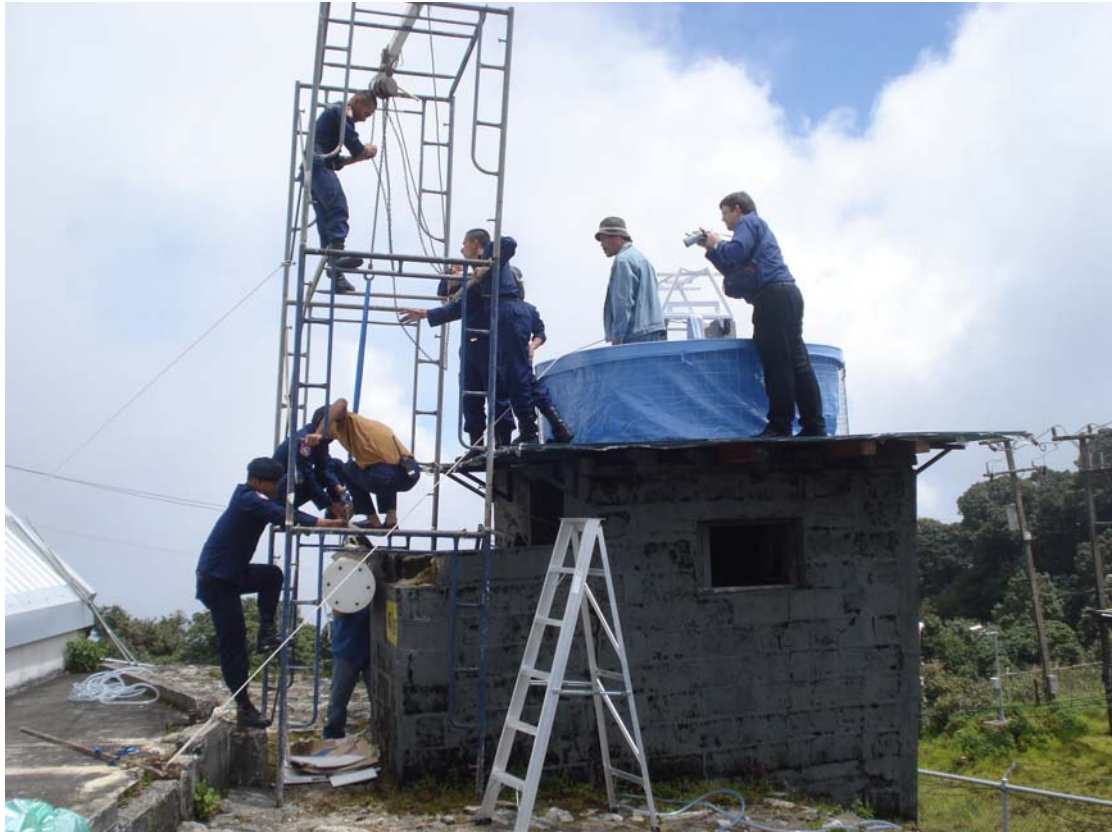
Figure 12: The calibration monitor (“calmon”) being installed at the summit of Doi Inthanon. The calmon is the white cylinder at the left. It is installed above a swimming pool so that the water provides a standard environment. The Principal Investigator is at the right, and a corner of the Princess Sirindhorn Neutron Monitor (PSNM) station is seen at the far left.
