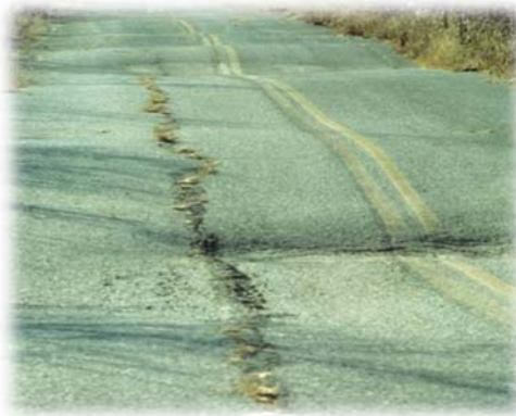
Fig. 4 Photograph showing road serviceability problem due to excessive differential settlement
