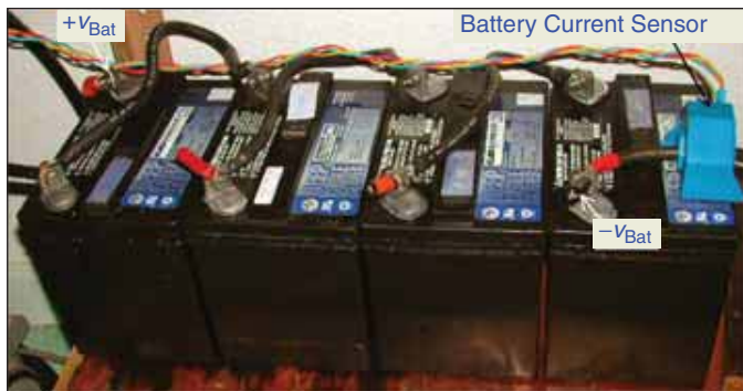
FIGURE 14 – Lead-acid battery module: 33 Ah and 48 V.
