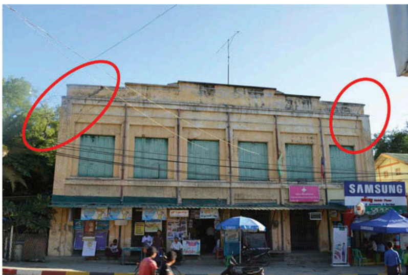
Figure 11. Moderate damage to unreinforced brick masonry building built during British colony era. The extensive shear cracking in the second story indicated that the façade was in an initial stage of failure.
