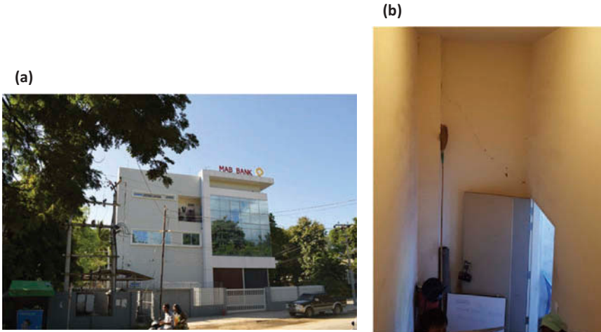
Figure 8. Light damage observed in reinforced concrete building in Chauk. (a) The vertical crack line occurred at the joint between main structure and concrete shaft causing pounding against each other during the earthquake and (b) observed in-plane shear cracking in URM infill. Depending on the wall geometry, in particular, the height/length aspect ratio, this URM infill is classified as flexural shear wall subjected to shear force and bending moment.
