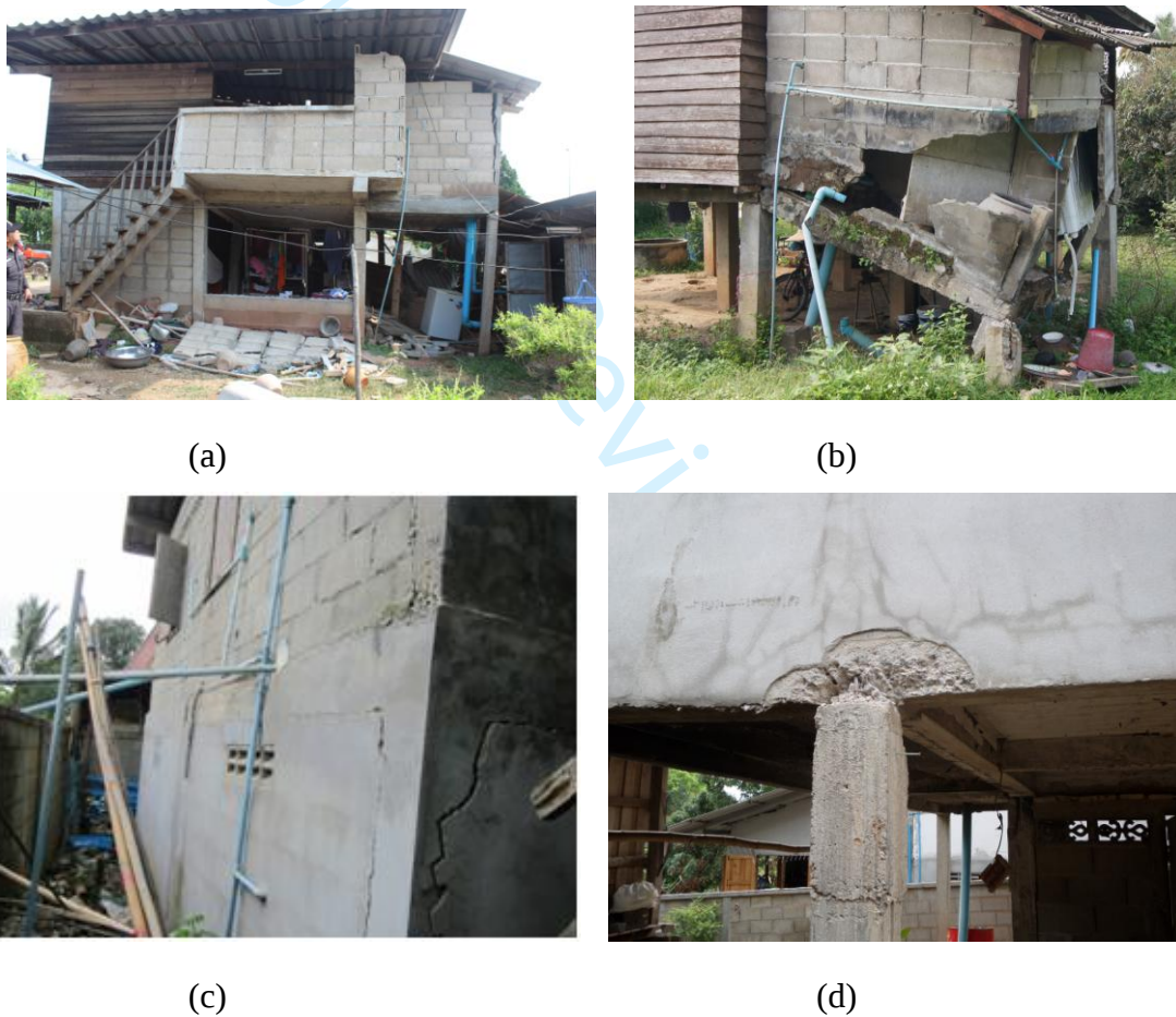
Figure 3 a). Typical seismic damage of building type II with partial or full failure of infill wall (red class damage), b) collapse of non-engineered column, c). Bending crack observed on infill wall (yellow class damage), d). Bending crack observed on non-engineered precast column (yellow class damage)
