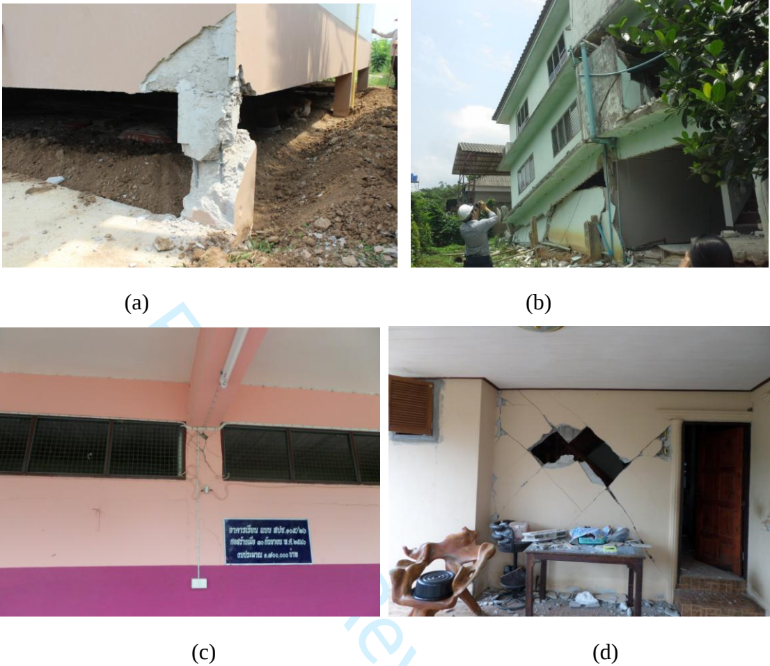
Figure 4 a). Short column failure of Type III structure b) soft story failure of 3 story RC frame (red class damage) c). Short column failure due to openings (yellow class damage) d). Diagonal crack observed on infill wall (yellow class damage)
