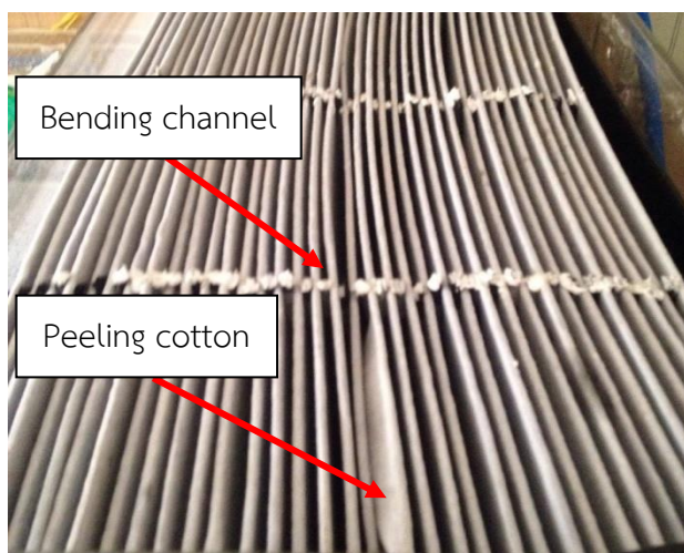
a. Former cooling core
