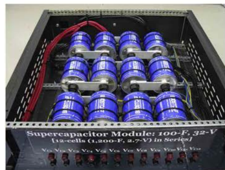
Fig. A2. Supercapacitor module (100 F, 32 V) used in the test bench.
