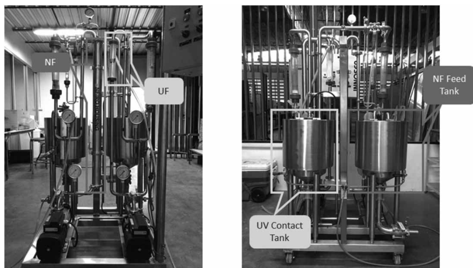
Figure 2 | The hybrid NF membrane and photocatalysis operation unit, showing the front of the unit (left) and the back of the unit (right).
